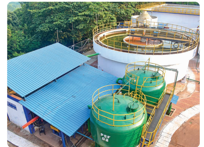
Water treatment plant at Noamundi, Jharkhand
