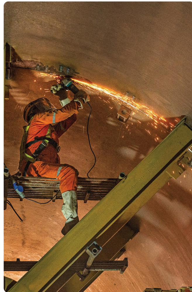
Blast Furnace, Tata Steel Kalinganagar Works
