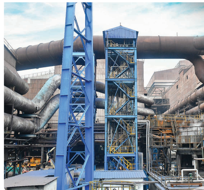
Commissioned India's first plant for CO 2 capture from Blast Furnace gas at Jamshedpur
